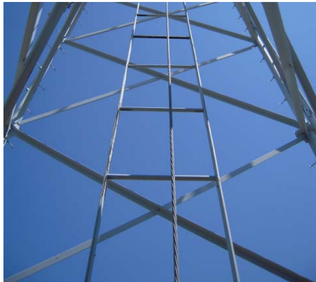
Photo 1-Tower Climbing Ladder with Safety-climb Cable
